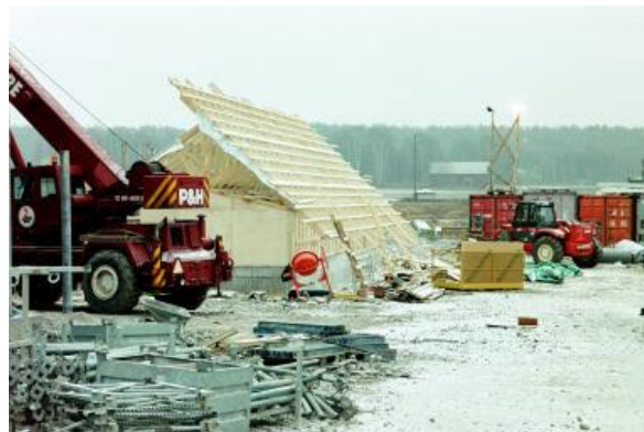
Fig.4. Construction site at Ekoviikki in late 1999. Upper picture shows the ATT(2) site in which 250 m 2 of collectors have been integrated into the house roof. The lower picture shows ATT(1) site and the collector support structure.
